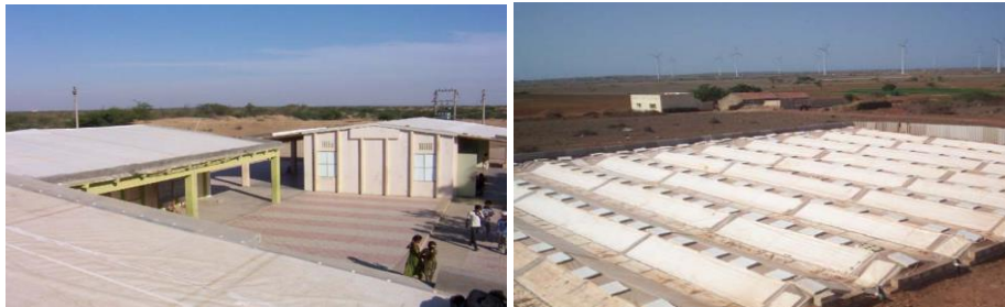
Figure 2. Condenser on Roof and Condenser on Ground, India
