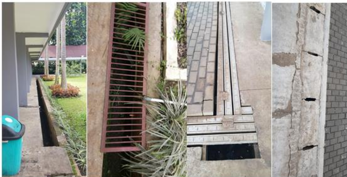
Gambar 3. Material penutup drainase di masjid Al-Furqan
