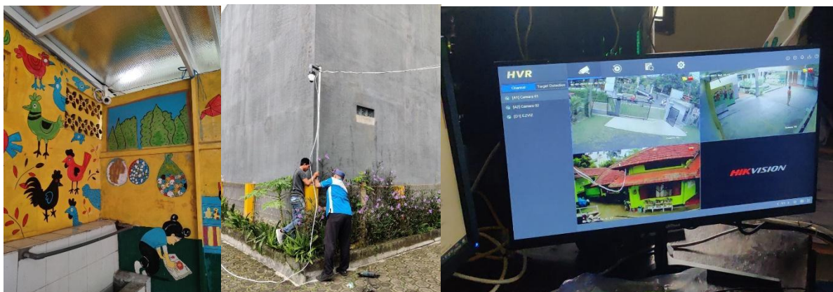
Figure 6. Result of CCTV installation and monitoring in real-time
