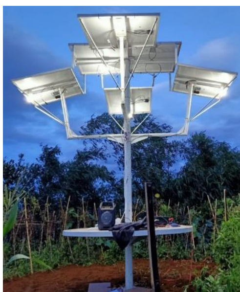
Figure 6. Solar Power Tree installed
