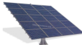
Figure 7. Solar Power Plant
