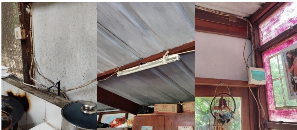
Figure 2. Existing Electrical Installation Conditions Before Revitalization
