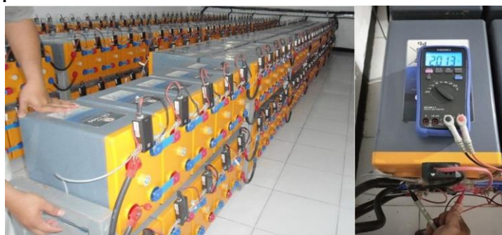
Figure 4. Checking the Battery Directly
