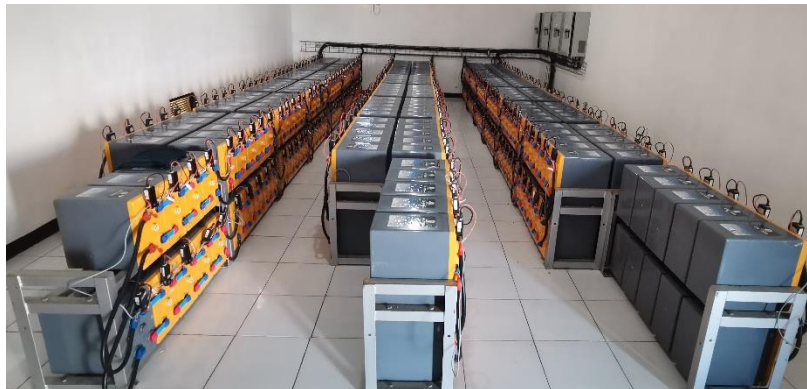
Figure 2. Storage Space Battery
