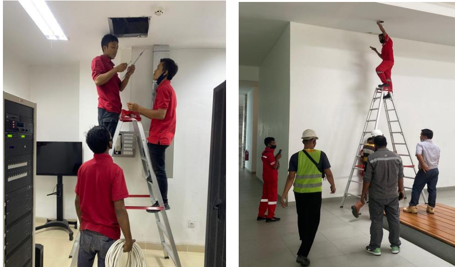
Figure 6. (a) Fire Alarm System Installation (b) Repair of The Sensor that Triggers The Alarm
