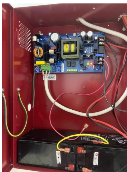
Figure 5. MCFA Backup Panel
