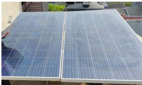
Gambar 5. Instalasi Panel Surya 600 Wp
