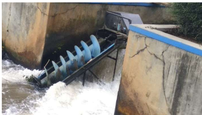
Gambar 7. Instalasi Mikrohidro Berbasis Turbin Screw
