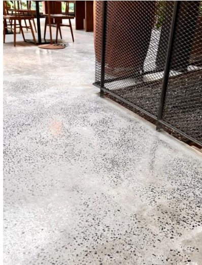
Gambar 2. Kondisi Lantai Ramu Kitchen
